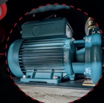
PUMP: External discharge pump
